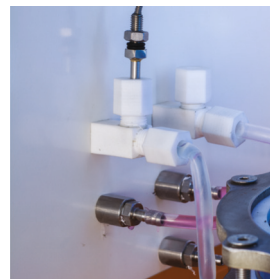
Live monitoring of input and output chiller temperatures
